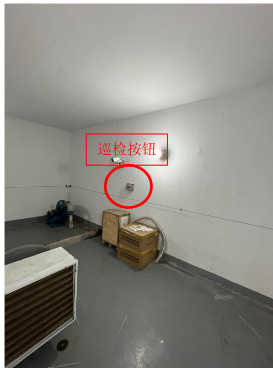
1#加速器机房主机室内巡检按钮
