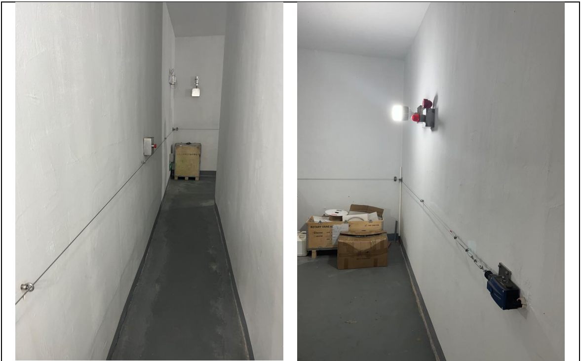
1#加速器机房主机室拉线开关
