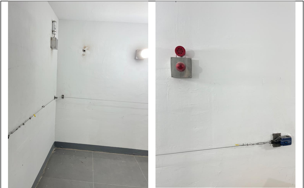
3#加速器机房主机室拉线开关
