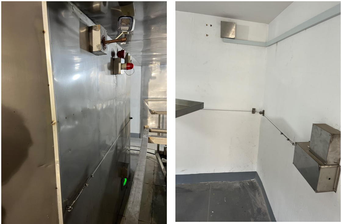
1#加速器机房辐照室拉线开关
