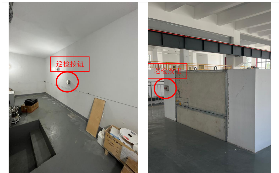
1#加速器机房主机室内巡检按钮
