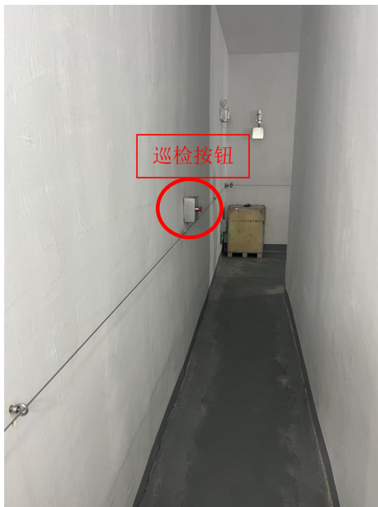
1#加速器机房主机室迷道巡检按钮
