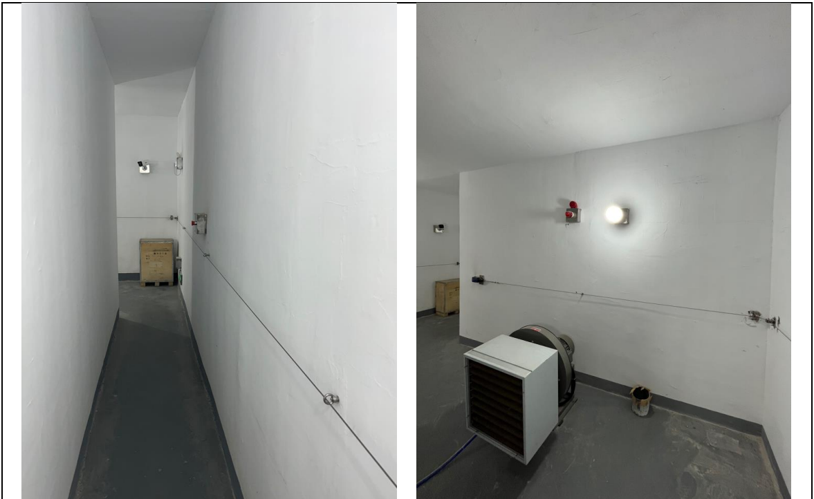
2#加速器机房主机室拉线开关
