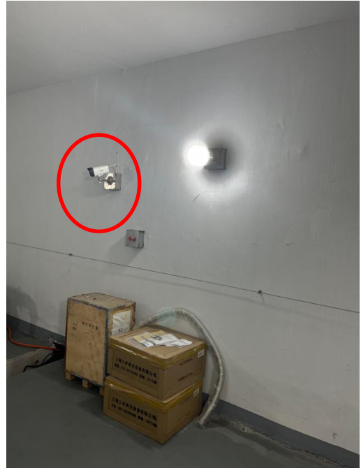
1#加速器机房主机室摄像头
